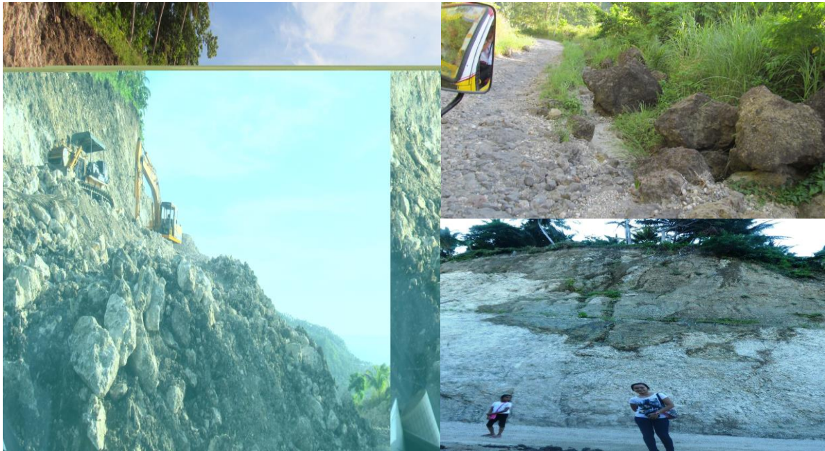
Figure 5. The road to Malayal is steep, hilly, narrow, and passes a mountain range that is vulnerable to landslide
